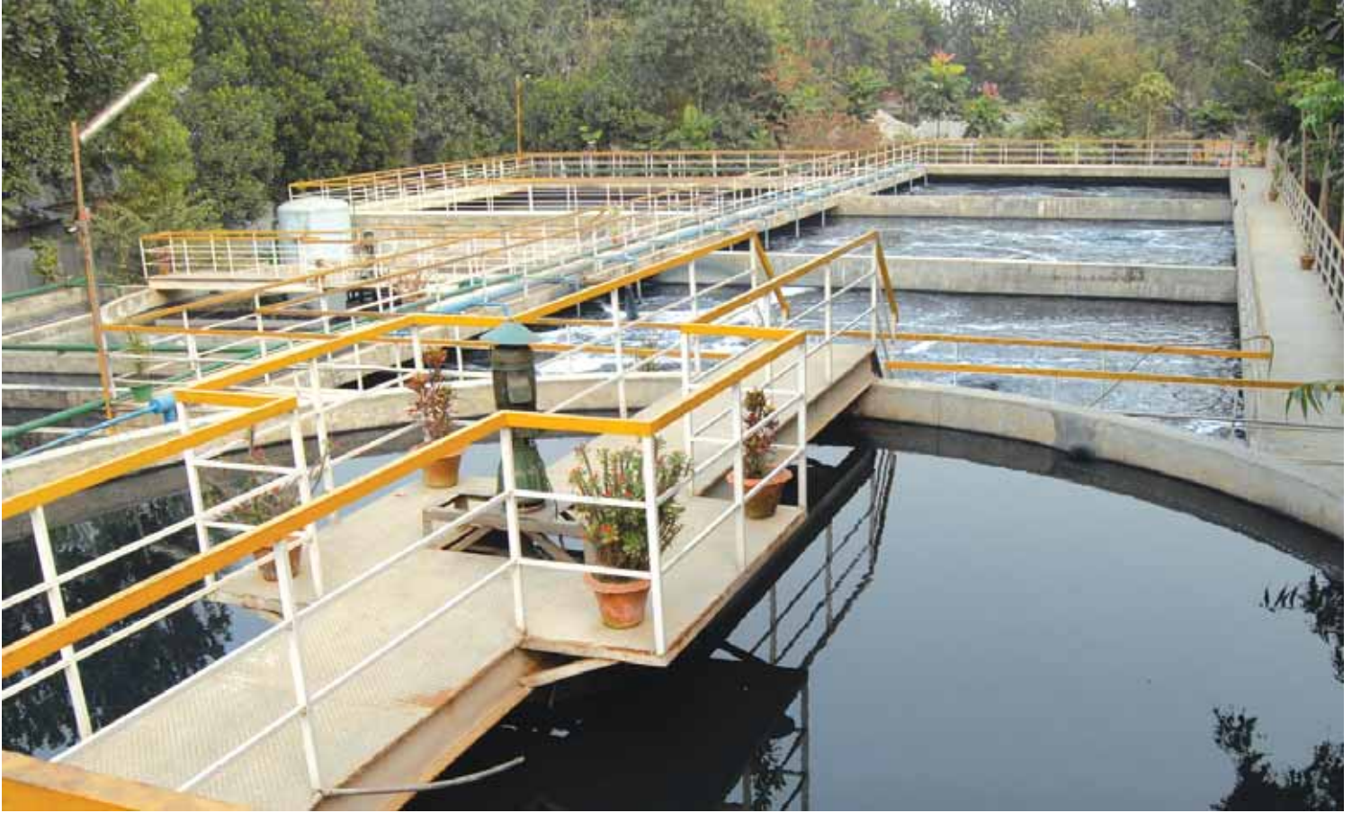
ETP, To help / protect environment by treating effluent.
